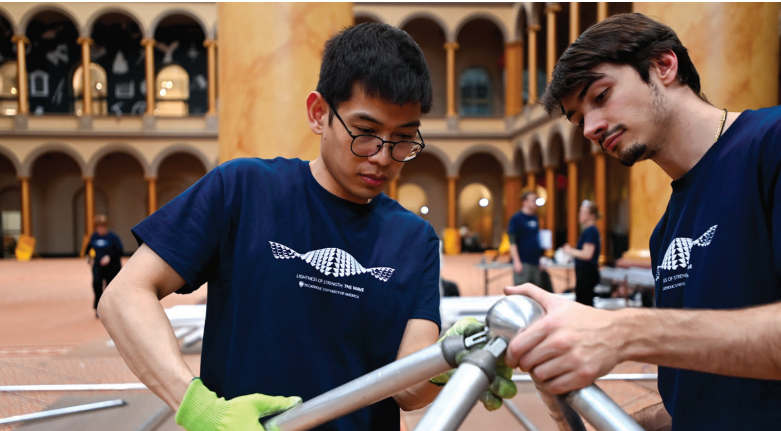
Students work on constructing "The Wave" in the National Building Museum's Great Hall. The 5,000-pound steel spaceframe was on display from Jan. 21 through Feb. 9, 2026.
